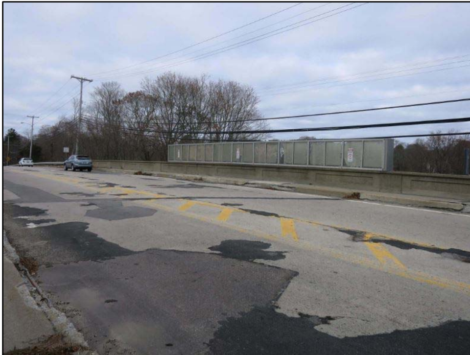
Figure 1-Poor Surface Roughness (Rating=1; IM=33%)
