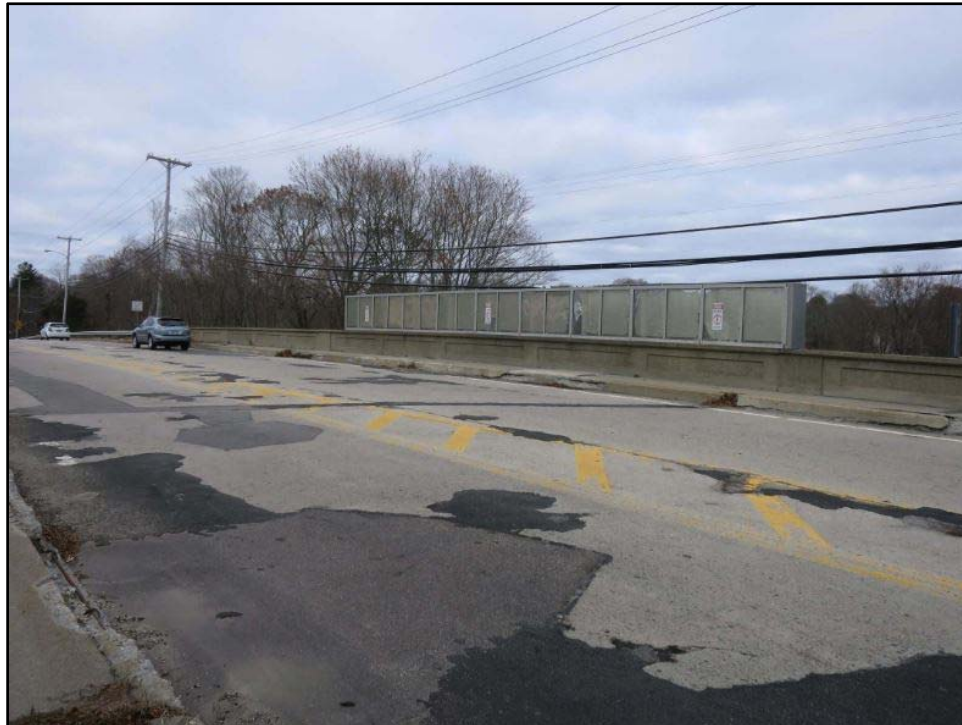
Figure 1-Poor Surface Roughness (Rating=1; IM=33%)
