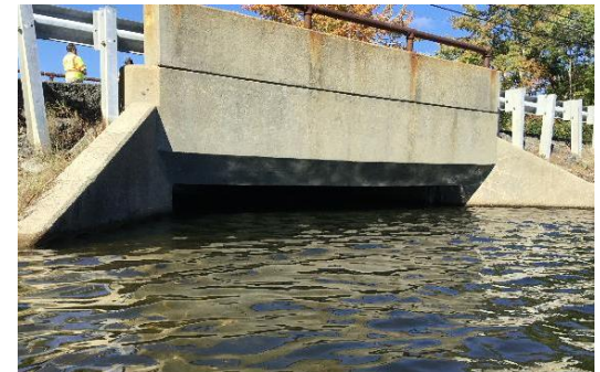
Example of undersized crossing
